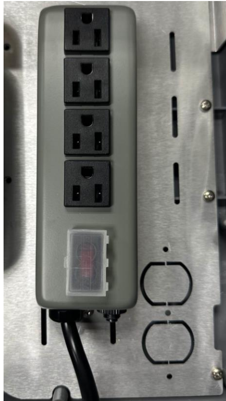
Figure 12: Power Strip Installation
