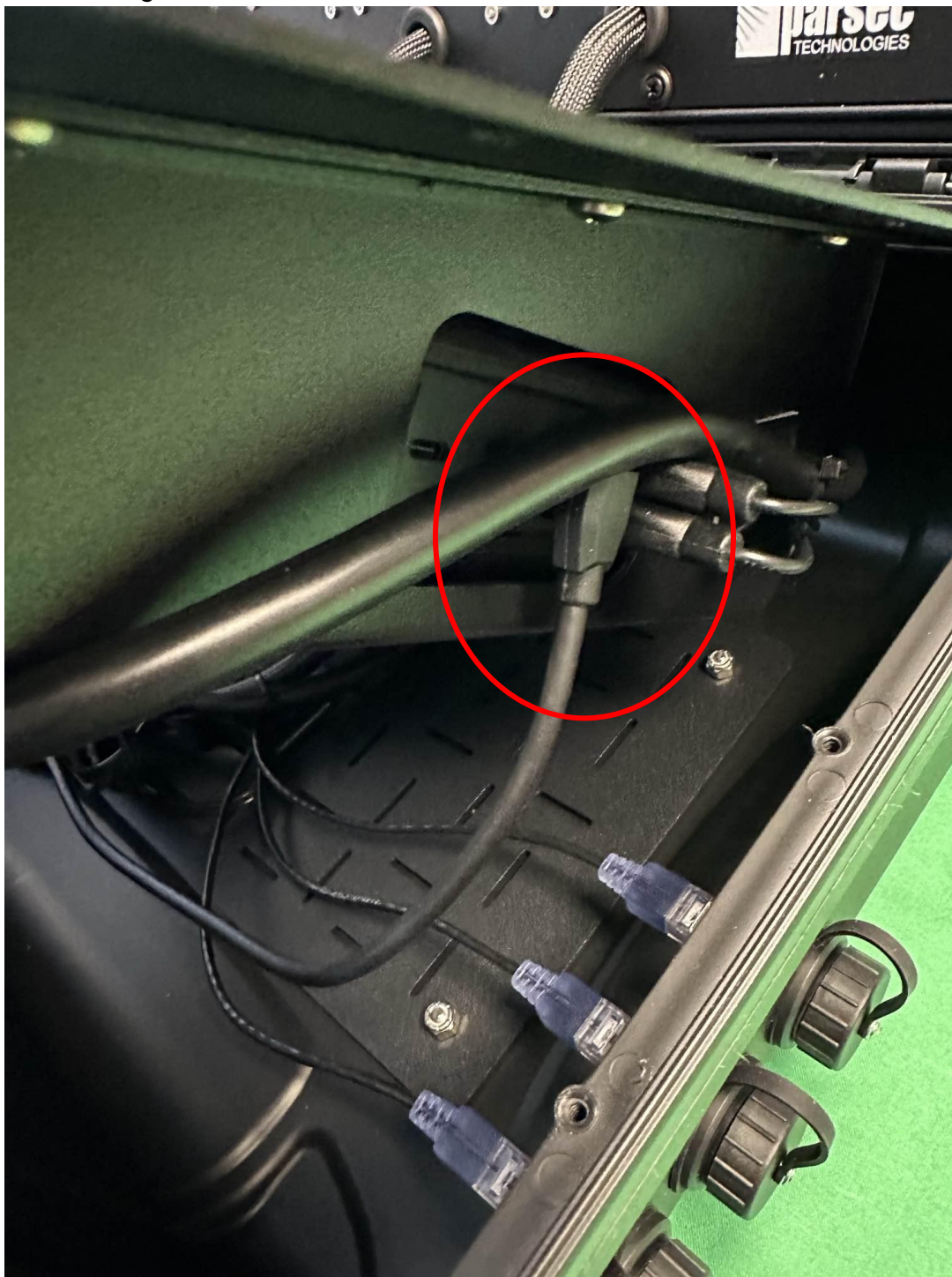
Figure 24: Charging cable connection
